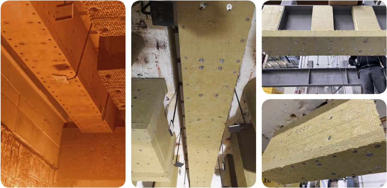
Fig. 5 Bottom slab with insulation thickness \geq 50 mm is fixed to the lower flange of the beam both with Fire Screws and welding pins.
